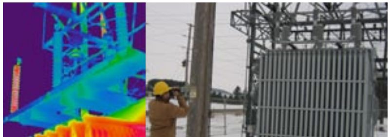
The infrared camera found this lightning arrester, shown on far left, indicating excess heat. The arrester was taken out of service before it caused an outage. Leadman/Technician Jeff Nelson uses an infrared camera at the Barron Substation to check the temperatures of equipment.
