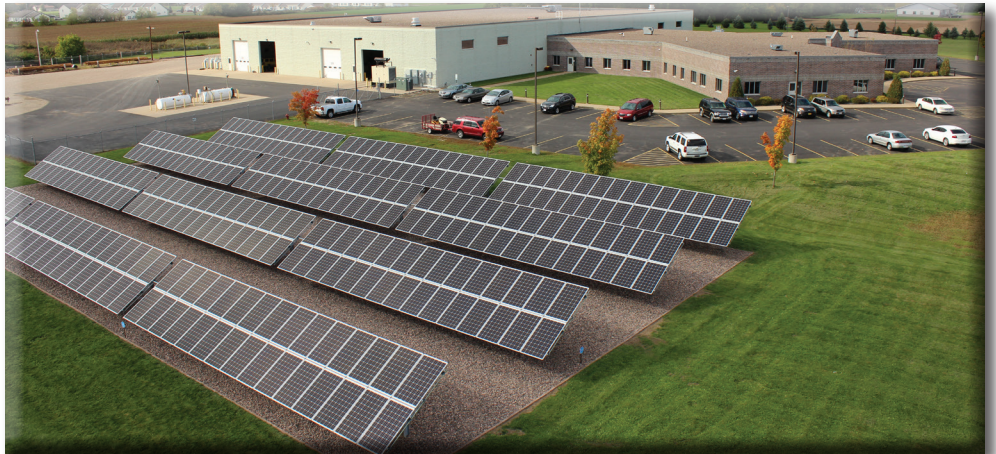
Community Rays was installed in 2014 at Barron Electric's headquarters and provides an affordable option for those members interested in purchasing renewable solar energy.
